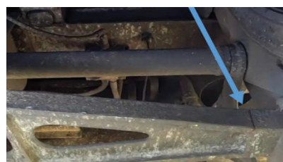
Fig. 15 Identification of defect Obr. 15 Identifikácia defektu
