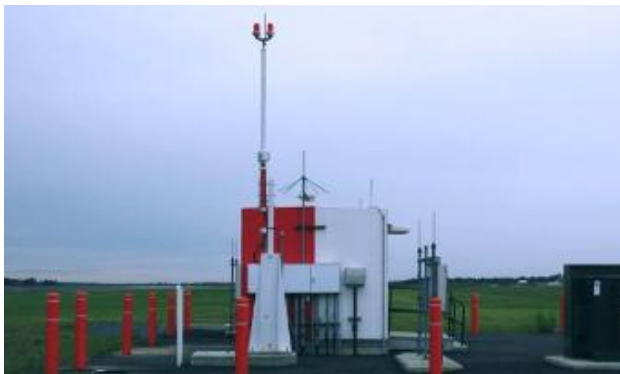
Figure 3. Distance Measuring Equipment
