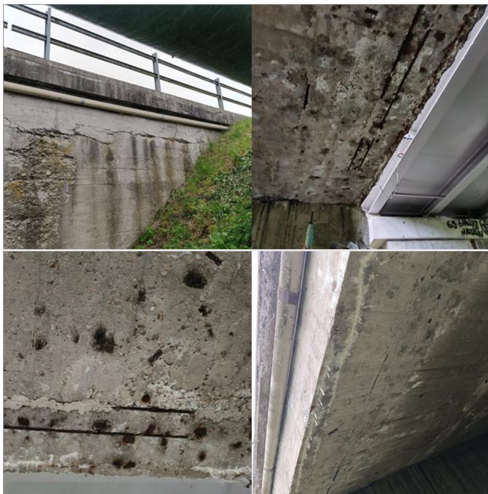
Figure 3 Defects on bridge M7441 (Figuli 2025)
